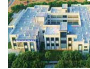
Civil maintenance work alongwith Fabrication and paint work of boundary wall of 'Smt. Mohini Devi Chachan Govt. College', Sahawa, Churu, Rajasthan.
