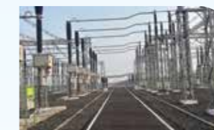
Transmission System in Rajgarh (BOOT)
